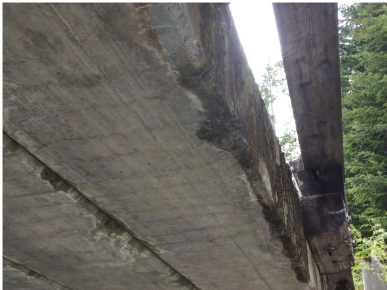
Damage noted to upstream slab
