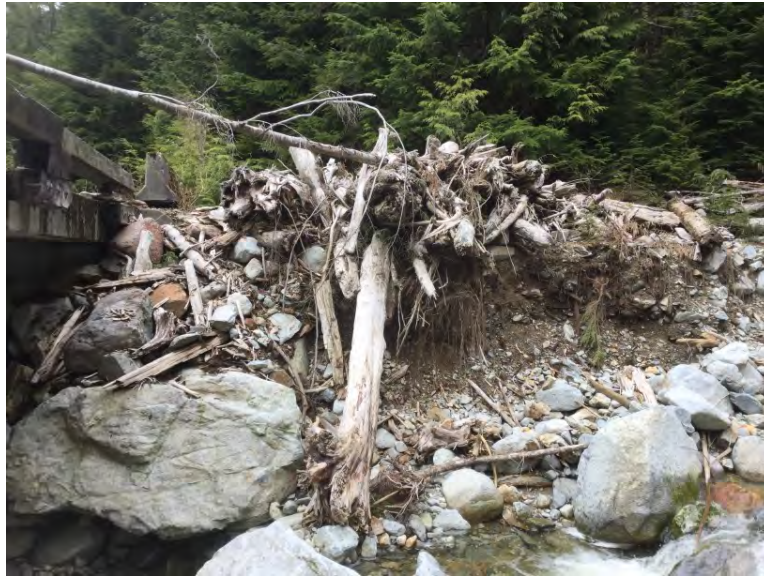
Debris accumulations at inlet
