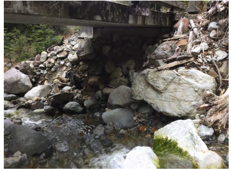
Riprap completely scoured at right abutment
